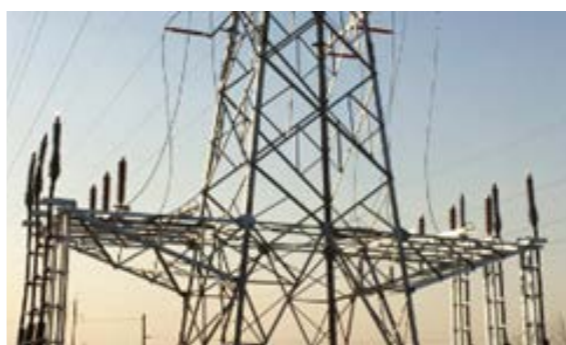
Linyi Electrical Seven Lines Lintai Project
