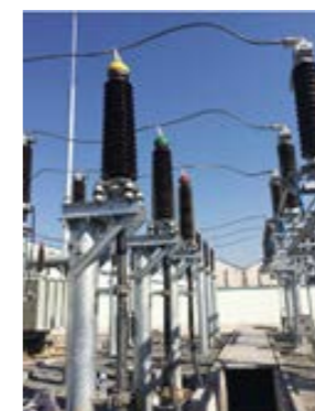
Guinea Keller Tower Power Transmission Project of Water Conservancy
