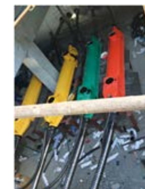
Argentine Interconnection of CTED -ET Dique-ET Tolosa HV transmission Line - 132kV
