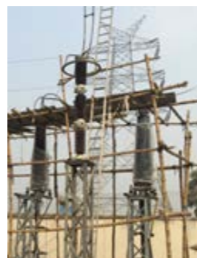
Bangladesh 78.50MW Gas Fired Rental Power Plant at GUORASAL BPOB
