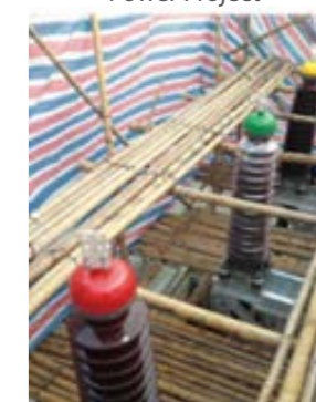
Jianhu County Xindian Variable Line Project
