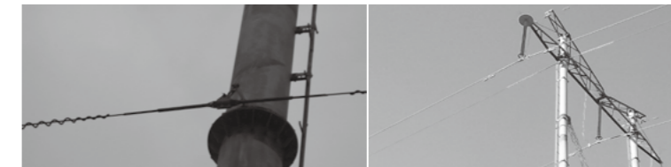
Installation on pole
